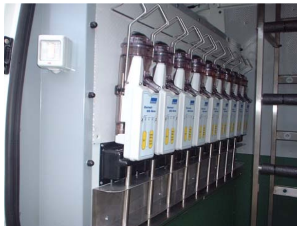
Inside of van showing a row of meters charging.
