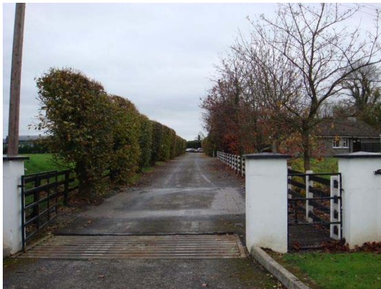
Wheel disinfectant bath to be built at Tully entrance. Edges cut but not yet excavated.
